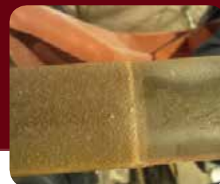
Boiler Tube After 2 Years Service
