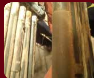
Boiler Tube After 2 Years Service
